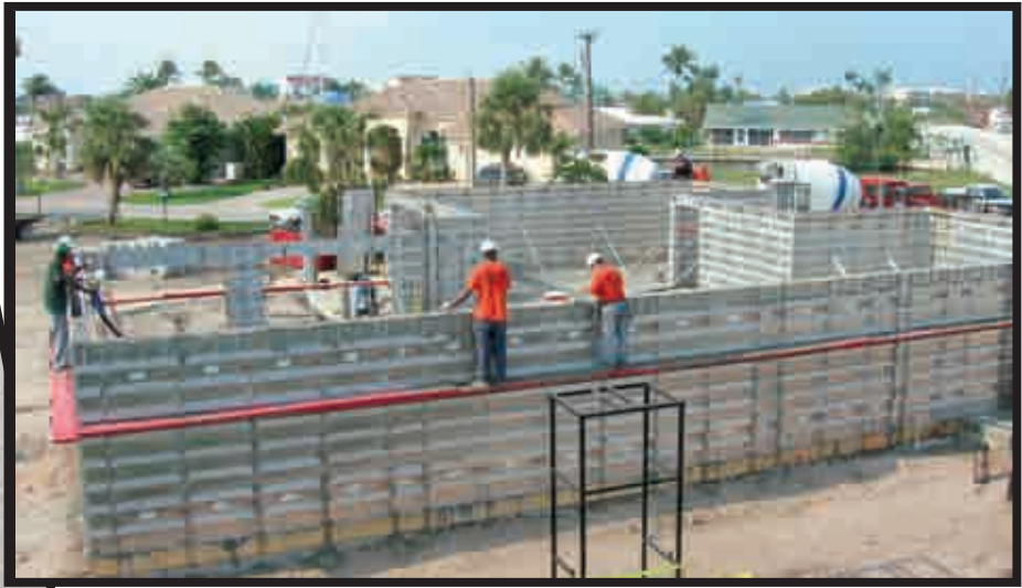
New windows and sliding doors are, of impact-resistant glass (left), and cast-in-place concrete walls (above) provide superior wind resistance and protection made from windborne debris.
