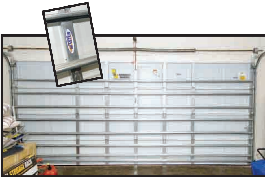
Eighty percent of residential hurricane wind damage begins with wind breaching garage doors, so an impact-resistant garage door is a must (above).
